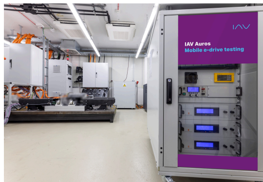
The IAV Auros Iso in the test facility.
